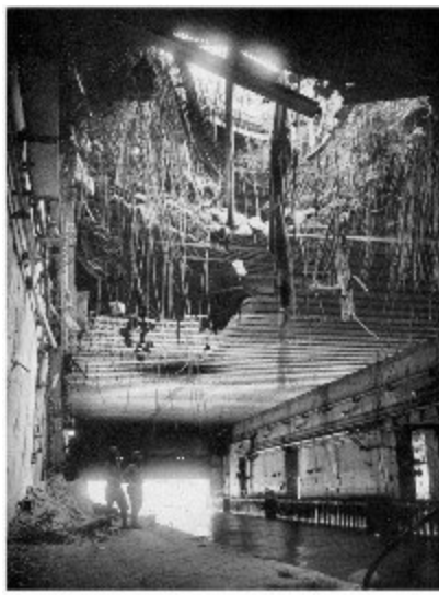
Bomb damage in a U-boat pen at Brest
